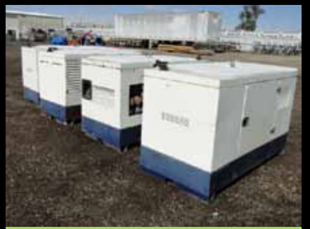
VIEW OF 2005 PRAMAC 30 KVA DIESEL GENERATORS
