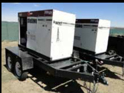
VIEW OF SHINDAIWA 70KW TOWABLE GENERATORS
