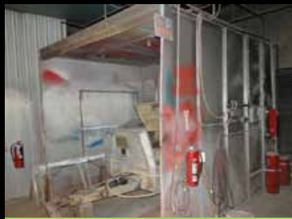
Paint Booth with Ansul Suppression System
